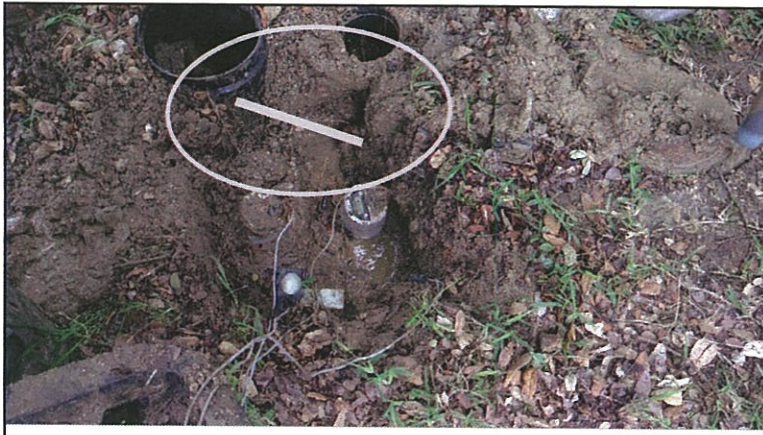
12 April 2018 – Approximate location of the iron utility cover discovered and removed by city water department personnel. Note the slot cut in the larger of the two valve boxes where the iron cover was inserted (presumably by either the water pipe/pavement contractor or city personnel installing the new water meters.
