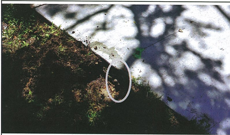
July 2018 – First leak discovered by Prolific Irrigation showing wooden stake presumably used by QROMEX to place concrete forms for the new portion of my driveway (with water turned off.)
