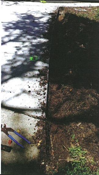
Area of irrigation leak excavated by Prolific Irrigation where they found the new driveway had been poured over top the existing irrigation line and sprinkler heads.
