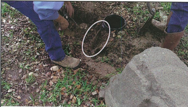
12 April 2018 – 10:35am. City Water Dept personnel discover iron utility cover inserted otop water line and 90 degree joints connecting water meter to my original line to 9622 Primrose home.
