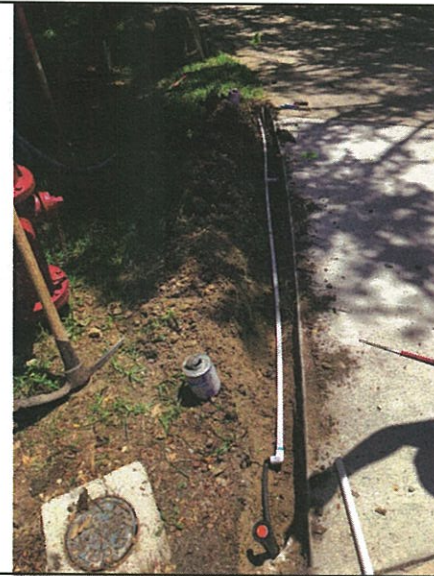
Area of irrigation leak replaced by Prolific Irrigation where they found the new driveway had been poured over top the existing irrigation line and sprinkler heads. Similar work was done on the other side of the driveway where the line and sprinkler heads were also damaged (adjacent to
