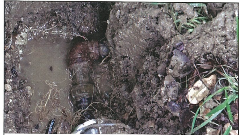
12 April 2018 – Closeup of one of two 90 degree fittings that the iron cover was directly touching.
