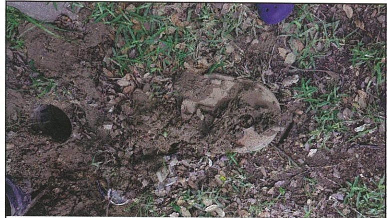
12 April 2018 – Iron utility cover laying flat after being removed by city personnel.
