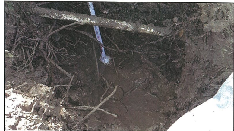
18 April 2018 – Tape measurer pointing to 45 degree fitting that was leaking (while water is turned off).
