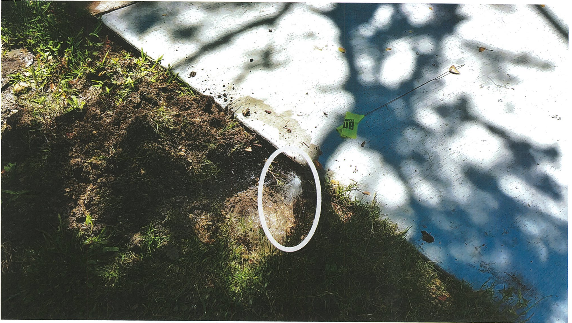
July 2018 – First leak discovered by Prolific Irrigation showing wooden stake presumably used by QROMEX to place concrete forms for the new portion of my driveway (with water turned on.)
