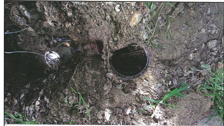
12 April 2018 – Closeup shot of work area and leaking 90 degree fittings.
