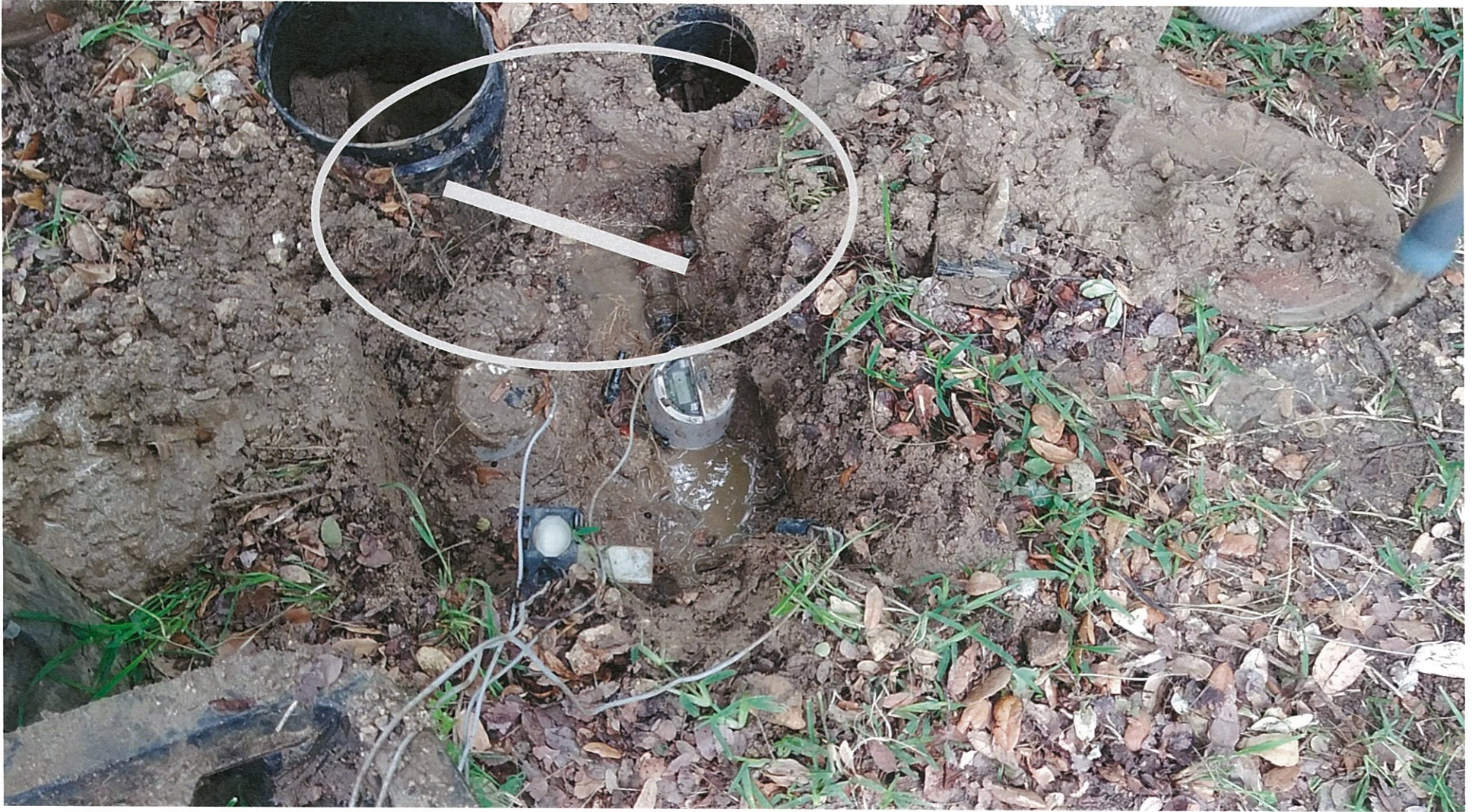
12 April 2018 – Approximate location of the iron utility cover discovered and removed by city water department personnel. Note the slot cut in the larger of the two valve boxes where the iron cover was inserted (presumably by either the water pipe/pavement contractor or city personnel installing the new water meters.
