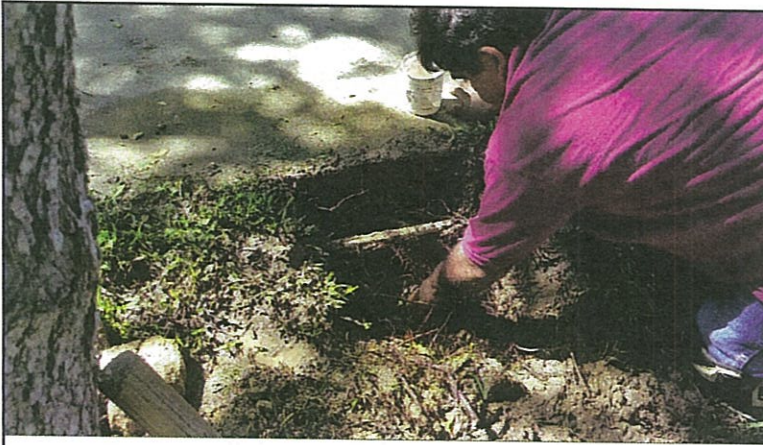
18 April 2018 – Discovered another leak further down the line toward my house (about three feet from the previous work, at the point the main water line goes under the slab. The 45 degree fitting (which I still have) was said by Bettencourt Plumbing to have been caused by excess pressure.
