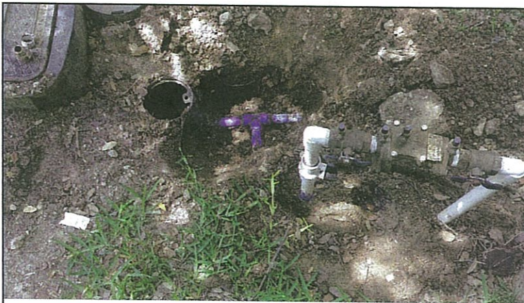
14 April 2018 – After my water softener exploded from excess pressure, Texas Blue Water excavated the original repair by the QROMEX contractor, showing absence of pressure reducing device originally installed there by Texas Blue Water.
