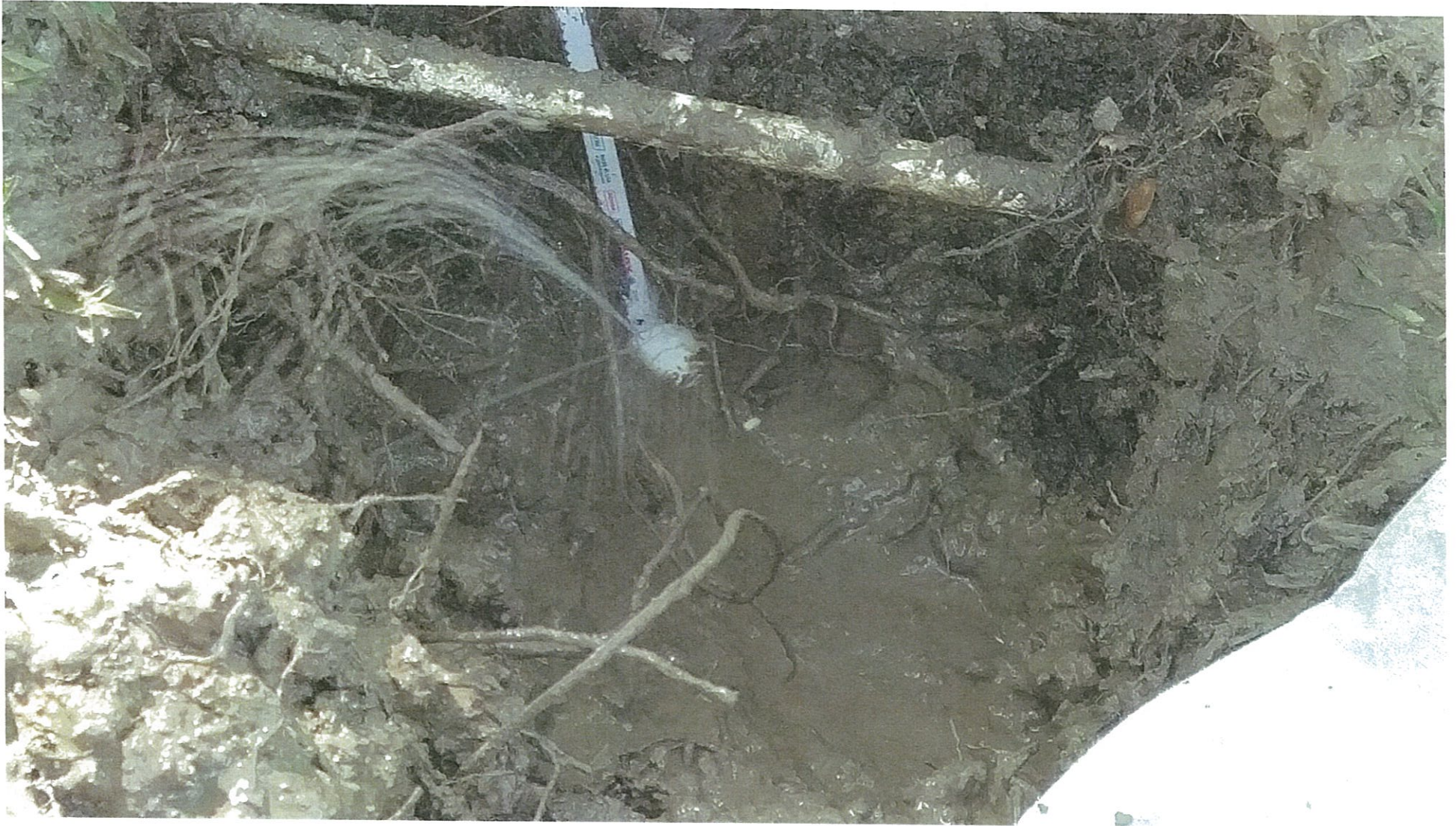
18 April 2018 – Tape measurer pointing to leading 45 degree fitting (after water is turned back on).
