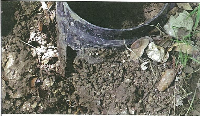
12 April 2018 – Clearer close-up of the cutout on the larger valve box where the iron cover was inserted vertically indicating it was intentionally placed in this position putting pressure on my water pipe and damaging the 90 degree fittings that were found to be leaking and later repaired by Immediate Response Plumbing.
