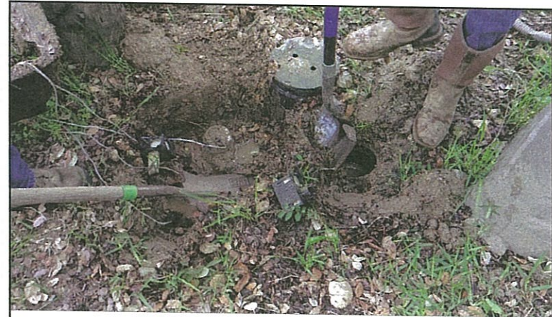
12 April 2018 – 10:35am. City Water Dept personnel digging out leak to determine which side of the meter the leak was on.
