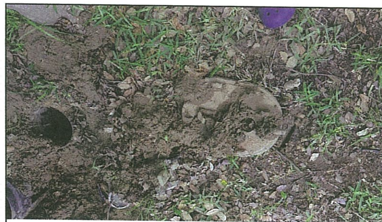
12 April 2018 – Iron utility cover laying flat after being removed by city personnel.
