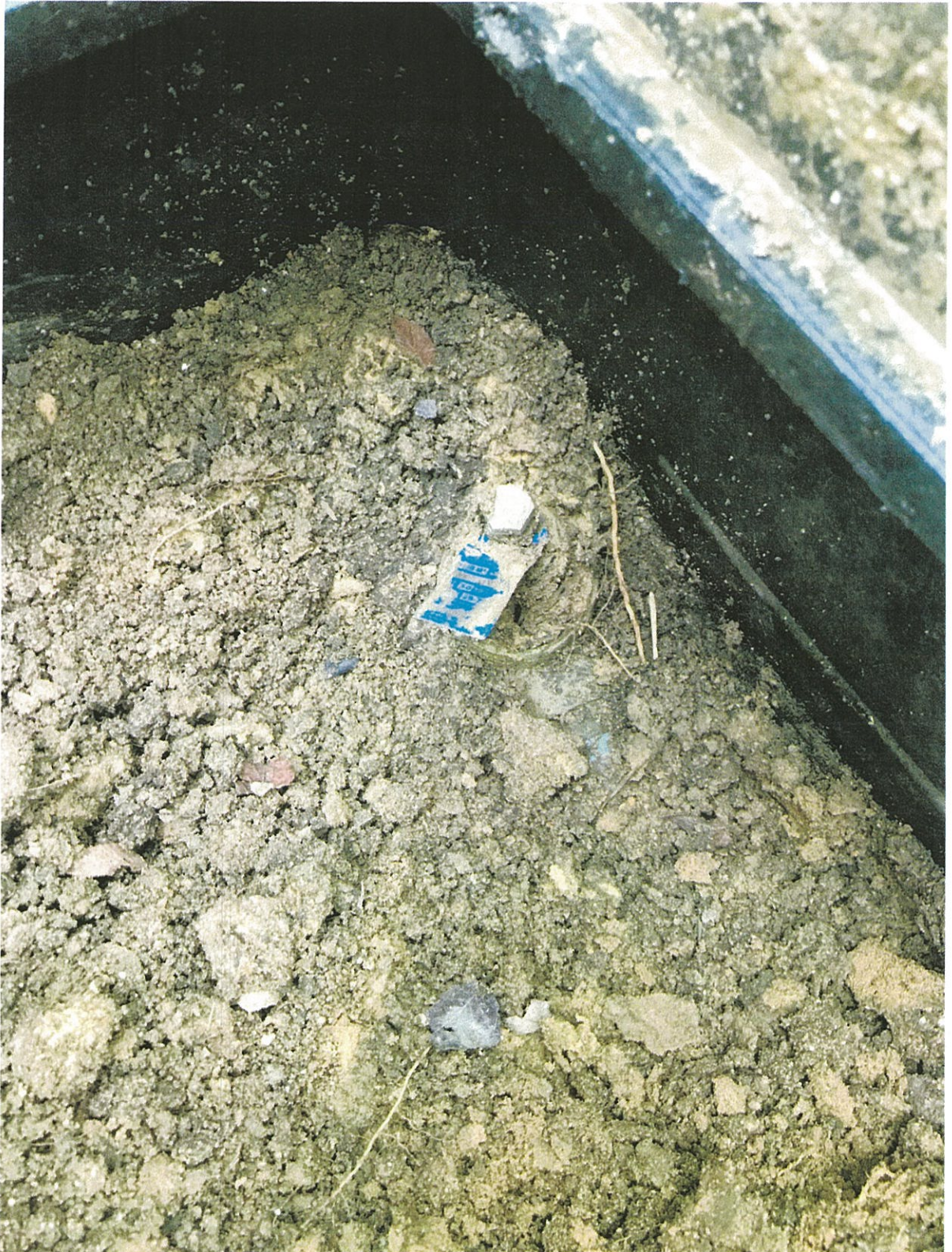
OLD PRESSURE REDUCING VALVE PHOTO #26
