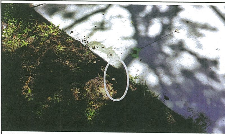
July 2018 – First leak discovered by Prolific Irrigation showing wooden stake presumably used by QROMEX to place concrete forms for the new portion of my driveway (with water turned off.)
