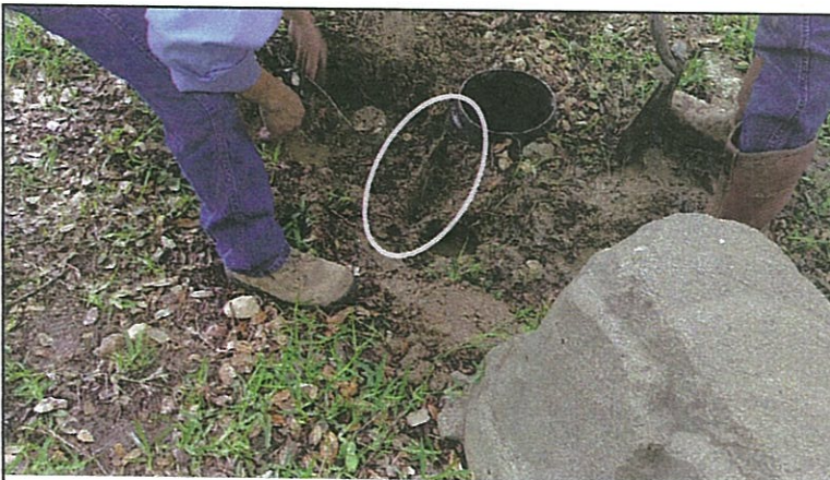
12 April 2018 – 10:35am. City Water Dept personnel discover iron utility cover inserted overtop water line and 90 degree joints connecting water meter to my original line to 9622 Primrose home.
