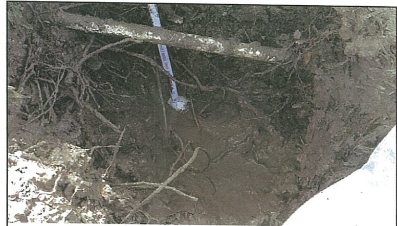
18 April 2018 – Tape measurer pointing to 45 degree fitting that was leaking (while water is turned off).
