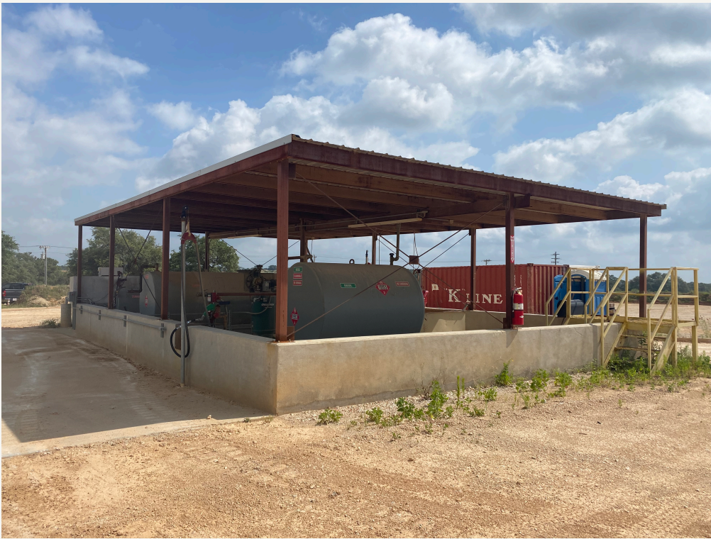
Fuel Containment Center
