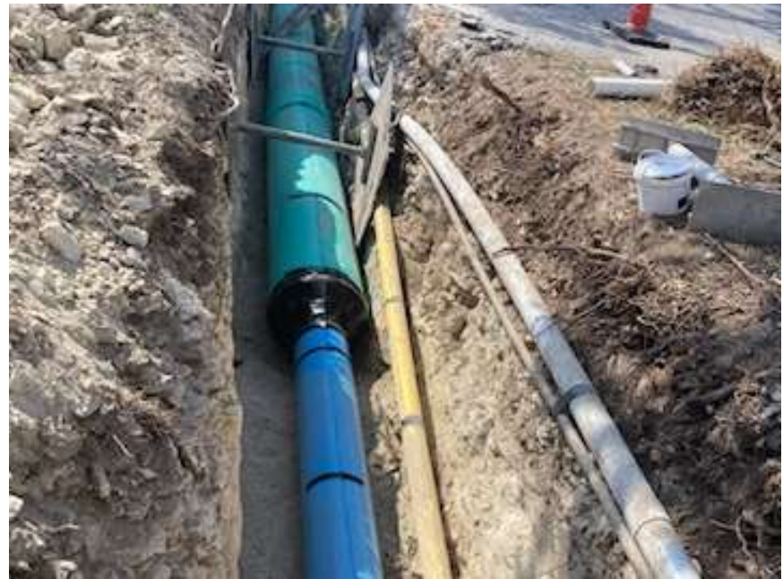
Encased Water Line
