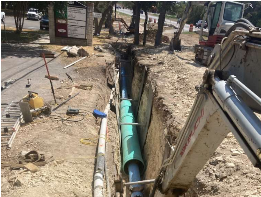
Encased Water Line
