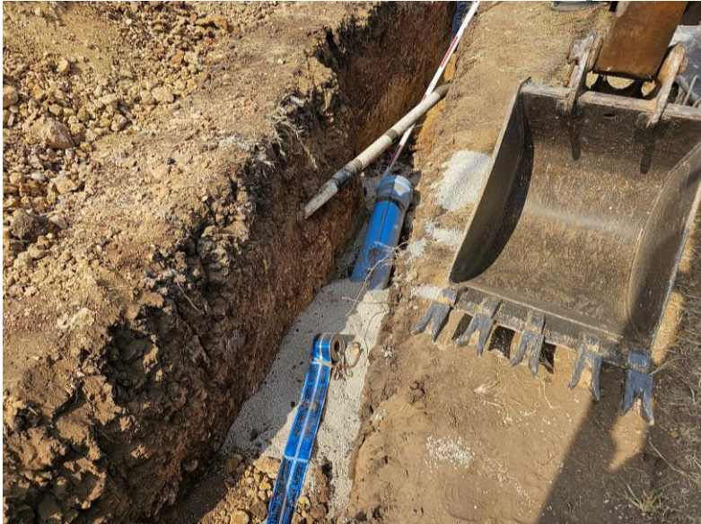
AT&T Utility Crossing
