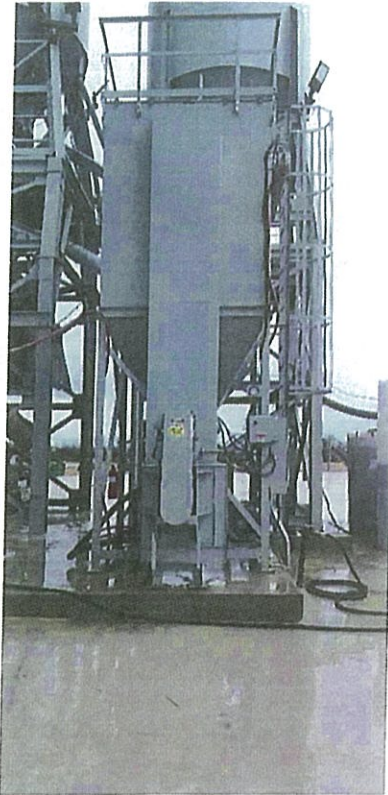
Photograph 01: Typical overview of centralized dust collector.
